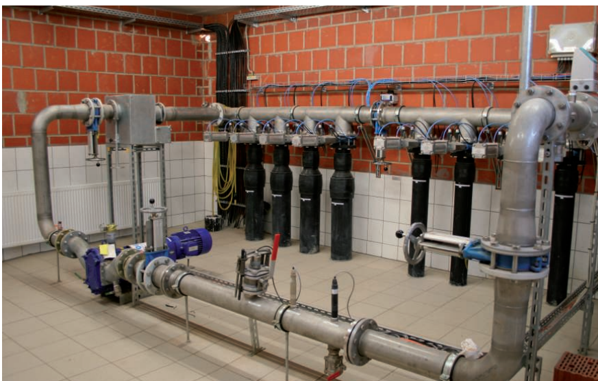
Fig. 3: Central pumping station of a biogas plant in Lelbach with online sensors (front)
