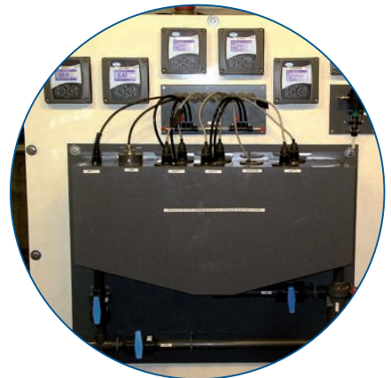
Fig. 5: Water quality monitoring station with digital controllers and sensor mounting
