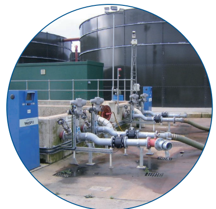
Multiple tanker stations
